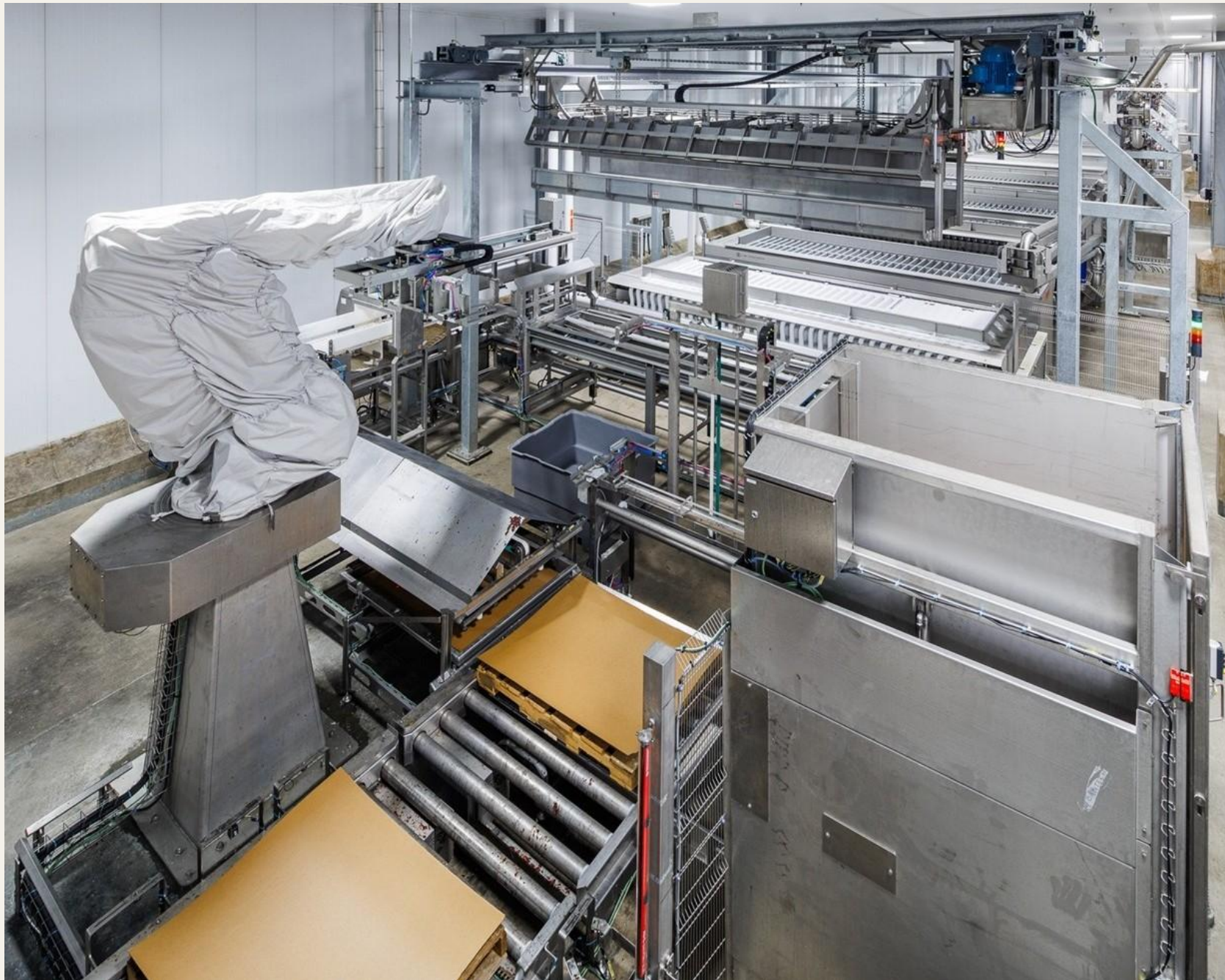
Shelby's new toll processing facility
